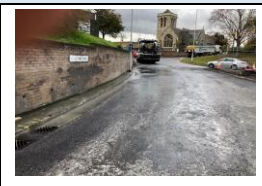
26th October - burst water main under the newly laid surface in Dover Street
