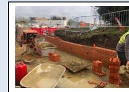
21st November - brick retaining wall being built at the junction of Station Street & St. Michaels Road
