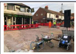
30th November (Phase 1 works) - block paving being installed on the table top in West Street
