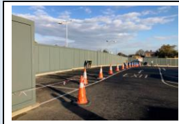
31st October - erection of the site hoarding around the Forum car park
