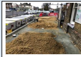
19th November - sand bed in preparation for paving in front of the station
