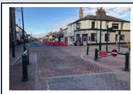
10th December (Phase 1 works) - block paving complete on the second table top in West Street
