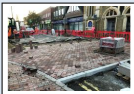
4th December (Phase 1 works) - block paving being installed to the second table top in West Street
