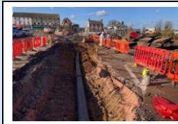
13th November - excavation in preparation for removal of the asbestos water main
