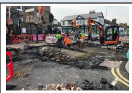
26th November (Phase 1 works) - excavation of the table top in West Street
