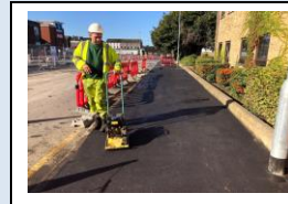
22nd October - surface course being completed on the footways ahead of the partial opening
